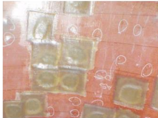
Figure 7.2: - Photograph of the inside surface of the inspected FRP tank showing features detected and characterized by the described standing microwave method
